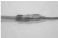
Orange wire connection
